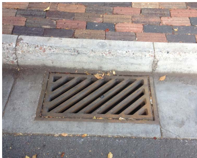
Figure 4.6 Grate Inlet used in City of Aspen
